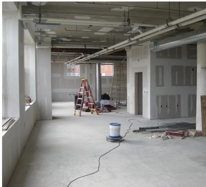
The third floor renovations will allow more space for students in the Media Collective as well as Woodworking & Furniture Design.
